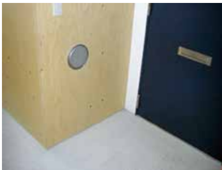
P.4. An Air-intake Register near the Entrance Door
