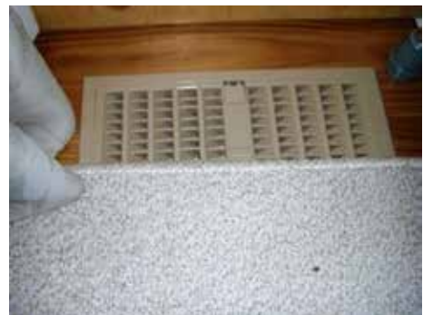
P.6. A Ventilation Register on the Floor of the Living Room
