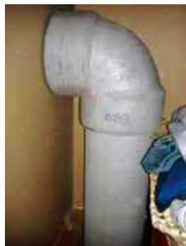
P.5. Ventilation Pipe to Heat Storage under the Floor
